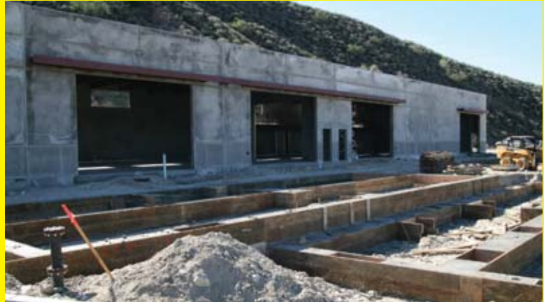
Scheduled for completion in late spring, the new Applied Technology Education Center (ATEC) located on the Canyon Country Campus will include five classrooms and approximately 10,000 square feet of workshop and laboratory space. COC programs slated to move into the ATEC upon its completion include a new solar energy technology program.
