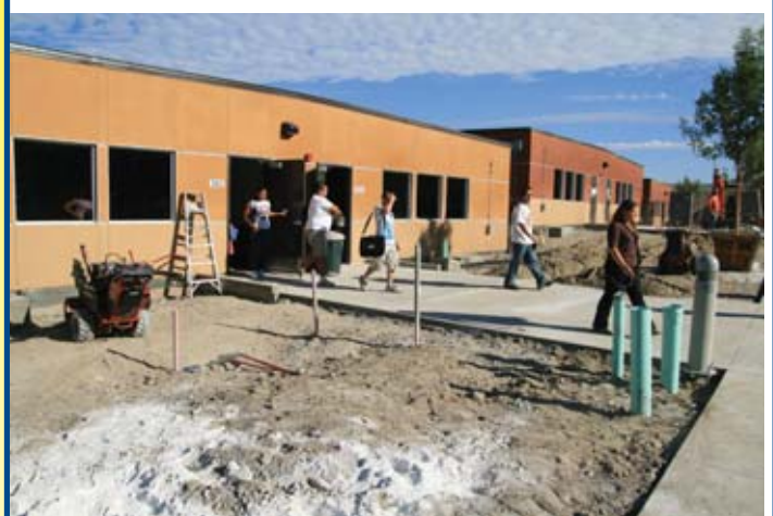
Students emerge from a modular classroom, at the still under construction COC Canyon Country campus, during the first day of classes back on August 27, 2007. At the time, the campus was still relatively unknown, as class sizes hovered at around 19 students.
