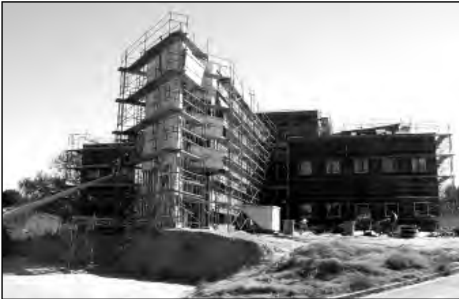
The Music-Dance Building has risen quickly and should be completed in early 2005.
