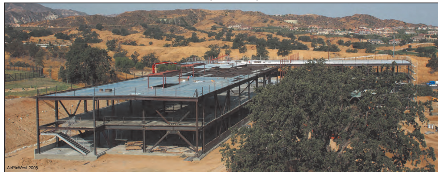
With the structure's major steelwork now finished, the 110,000 square-foot Dr. Dianne G. Van Hook University Center is scheduled for completion by April 2009. Located on the southern boundary of COC's Valencia Campus, the $38 million building will house up to 10 partner universities and offer more than 70 degree and credential programs from schools including UCLA, Chapman University and both CSU Bakersfield and Northridge.
