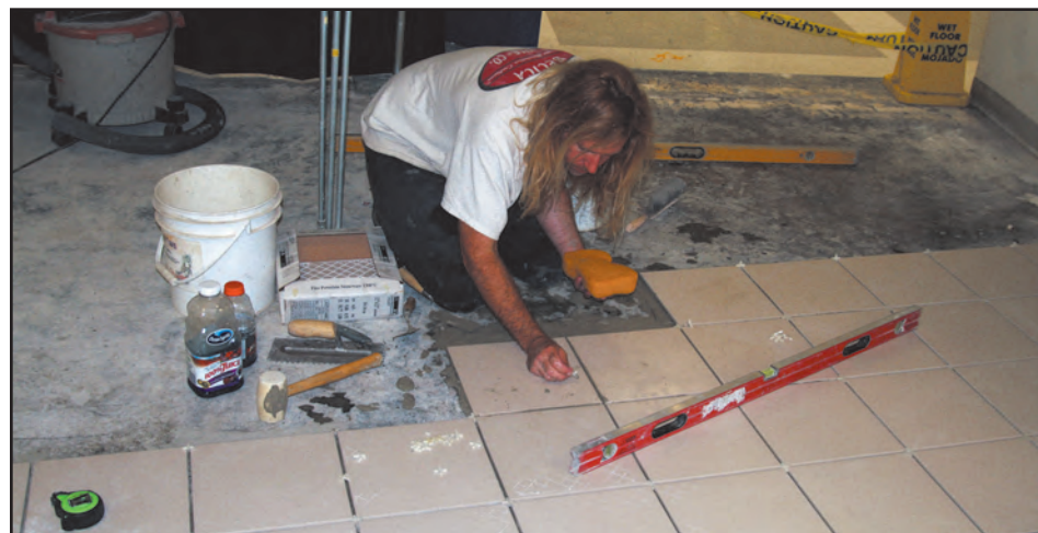
New floor tiles are being installed as part of a major cafeteria renovation that will include a Culinary Arts teaching kitchen.
