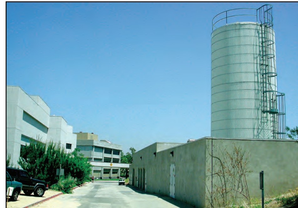
College of the Canyons uses several central plants, such as this one near the library, to provide heat, air conditioning, and both hot and cold water in an energy-efficient manner.
