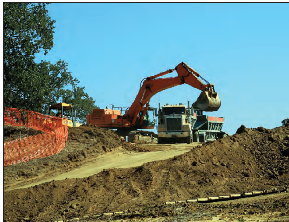
Site preparation has begun for the Dr. Dianne G. Van Hook University Center, which will house degree programs from an assortment of public and private universities.
