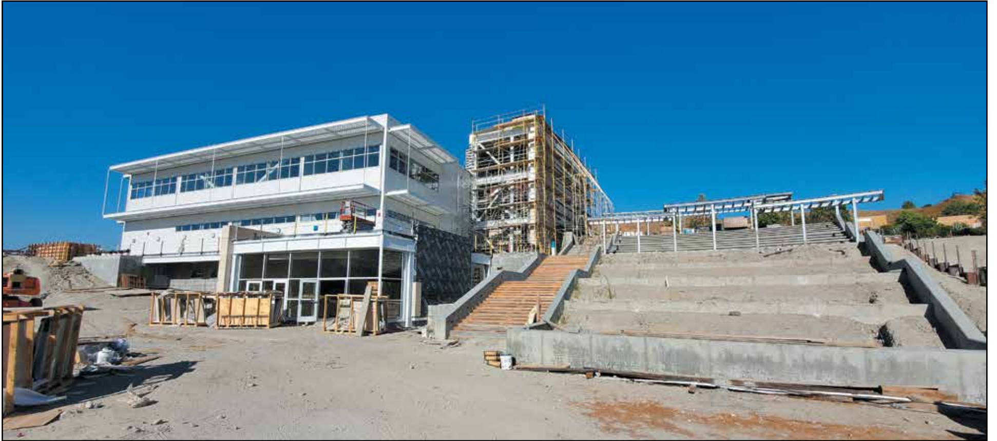
Construction of the Science Center at the Canyon Country campus is on track for completion later this year. The center is expected to open for instruction next summer.
